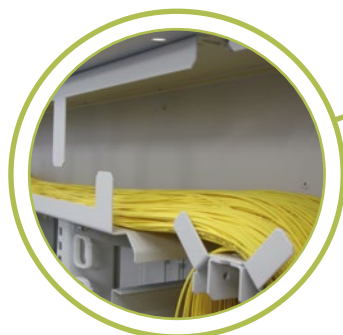
Horizontal communication cable raceways between juxtaposed distribution frames
