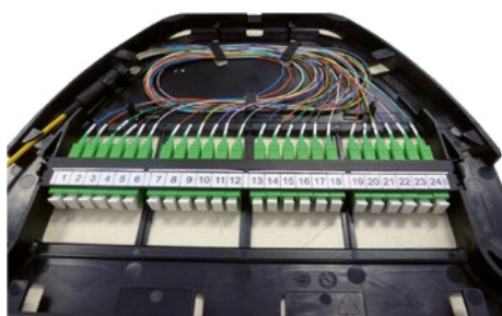
Example of a connection in an iTOM-V3 rack
