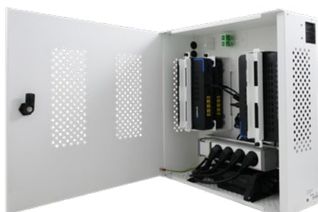
Perforated door providing protection and ventilation for equipment
