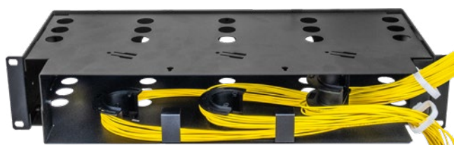
Patch cords overlength management coming from the right
